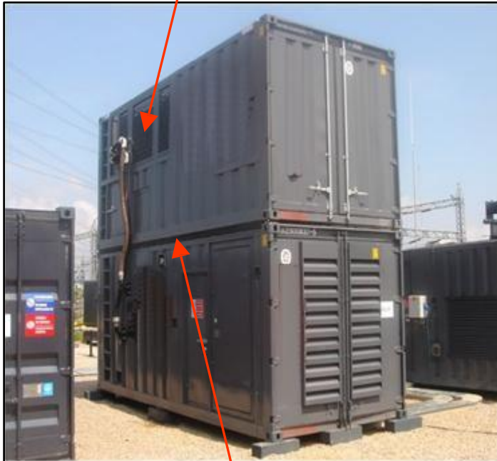
Air intake louvers for LT cooling coils
