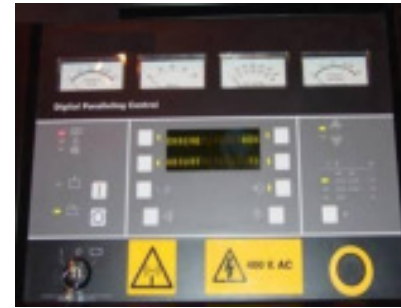
Power Command Control
